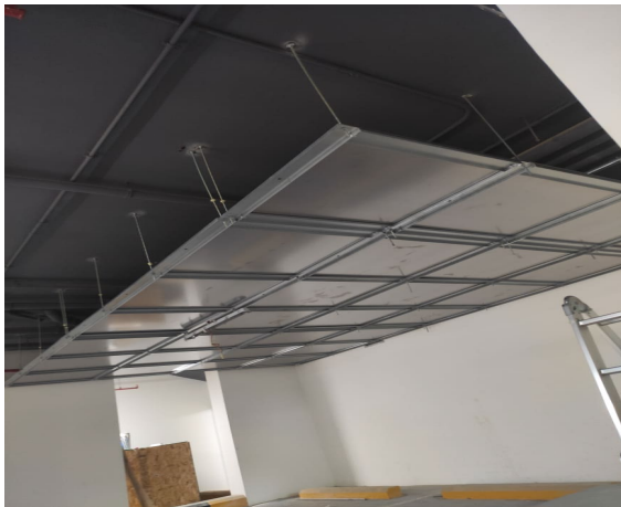
Image 5: Magnetic Shielding Below the MRI Room.
